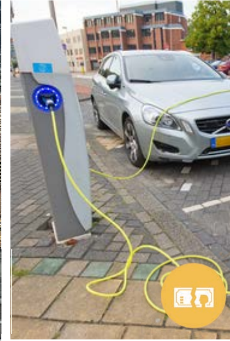
Rotterdam EV- charging point
