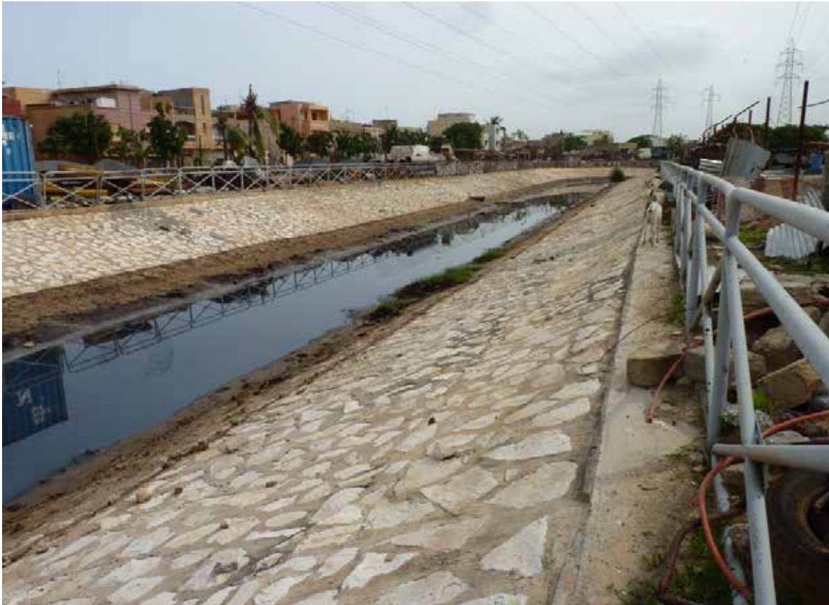
A drainage channel, at Dalifort-Foirail, allowing rainwater to flow towards the sea.
