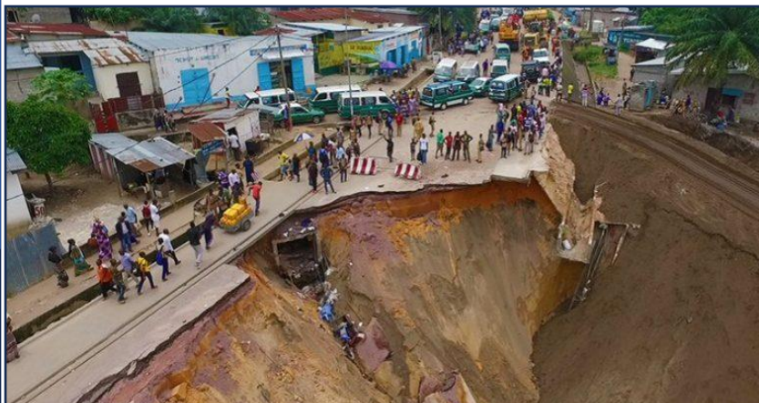
Erosion de la route de Ngamakosso (source: ADIAC)
