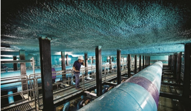
Unique Ice Thermal Storage System
