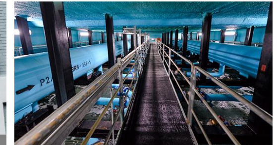
District Cooling System (energy and water – chiller)
